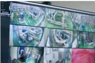
① Control of major facilities and fire monitoring
