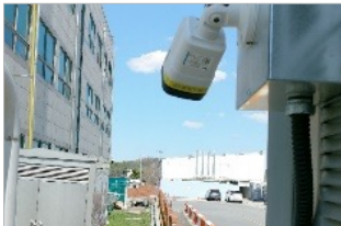
⑤ Perimeter control
